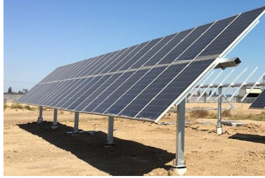
Figure 1: Single-Axis Solar Tracking Systems
