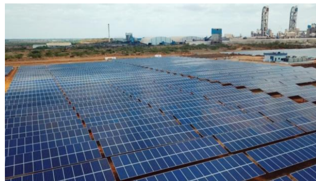
Figure 4: 10 MW Ground-Mounted PV Plant at SCCL, Jaipur, Telangana.
