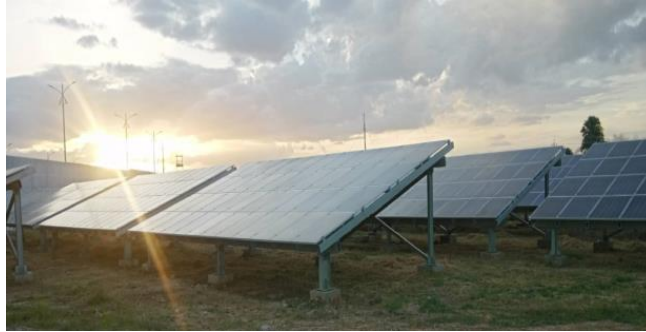
Figure 2: Ground-Mounted PV Plant at JNTUH, Sultanpur, Telangana.
