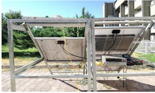
Figure 6. Back view of photovoltaic systems
