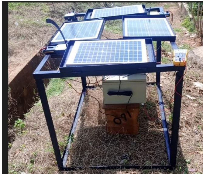
Figure 1: Experimental setup showing the PV modules, charge controllers, batteries, and measurement instruments installed at Auchi Polytechnic.
